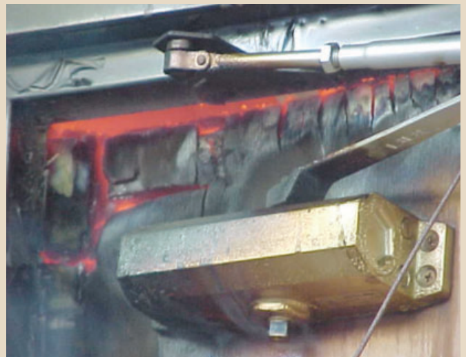
A photo of the head of a door which has not failed integrity according to the 150 x 6mm continuous gap failure criteria but which would provide excessive smoke leakage
